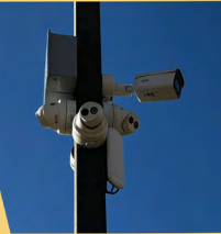
32 Security cameras in Education wing, Life Center, and parking lot
